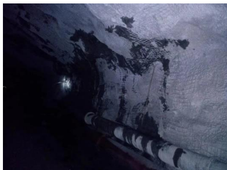
Fig. 5 Fracture migration and water seepage in surrounding rock of fracturing roadway
