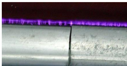
Figure 1. corona discharge in 1000kV UHV transmission project
