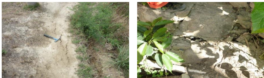
Fig. 1 2#Landslide deposit on the western edge cracks
