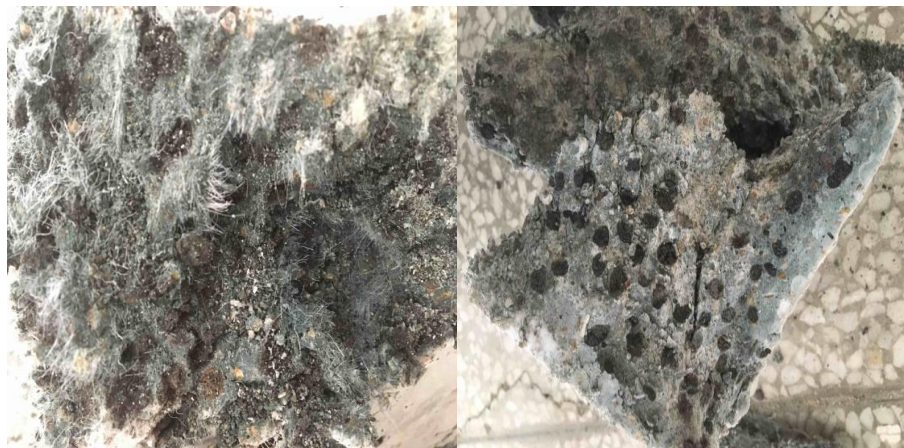
Fig. 2 the damage sketch about ceramsite concrete
